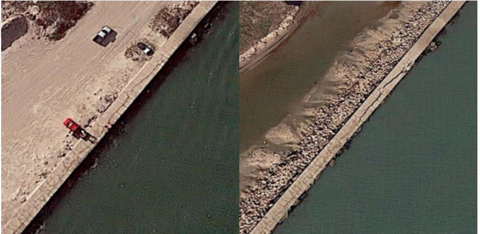
Comparison of pre- and post-satellite imagery suggests a failure crack is present in the seawall along the southern side of the Aransas Pass.
