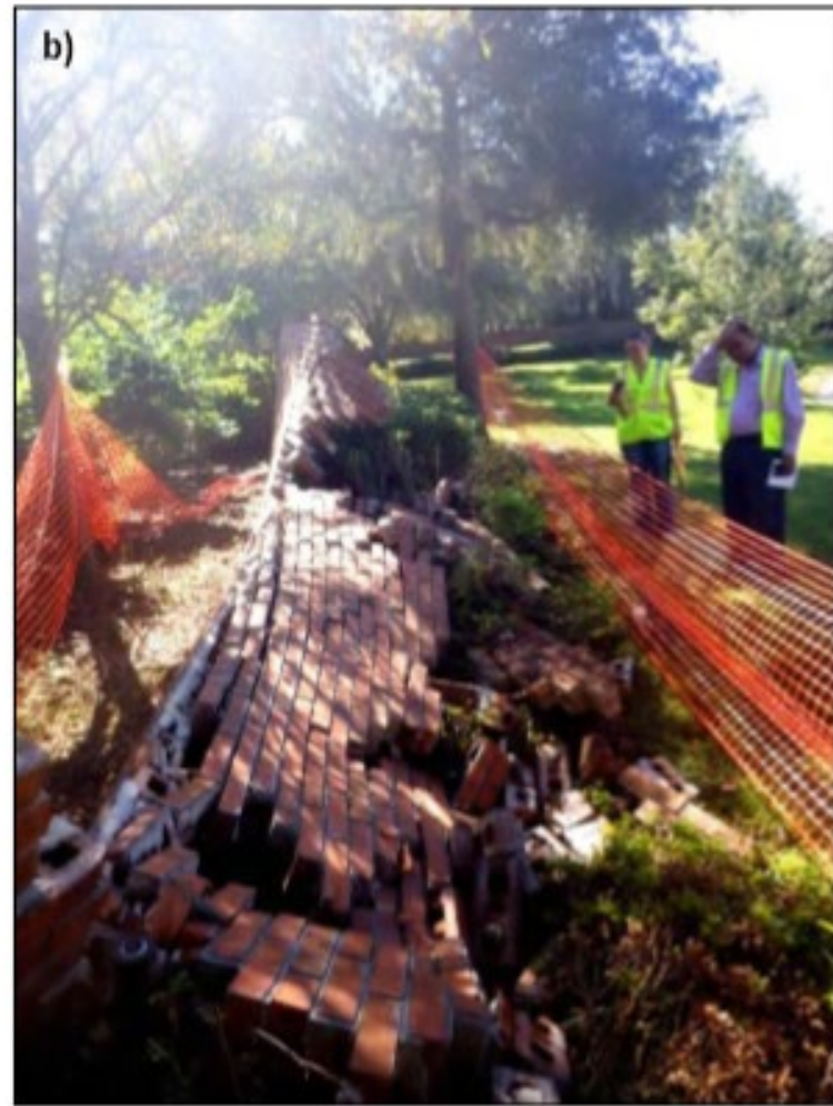
The erosion in the retention pond during the hurricane and the 12.5 meter length brick wall was toppled at sinkhole E
